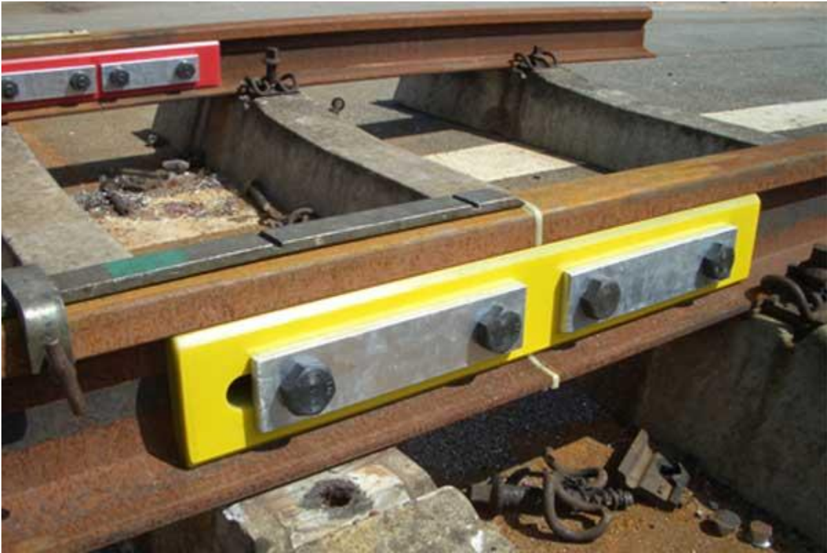
Insulated rail joint
